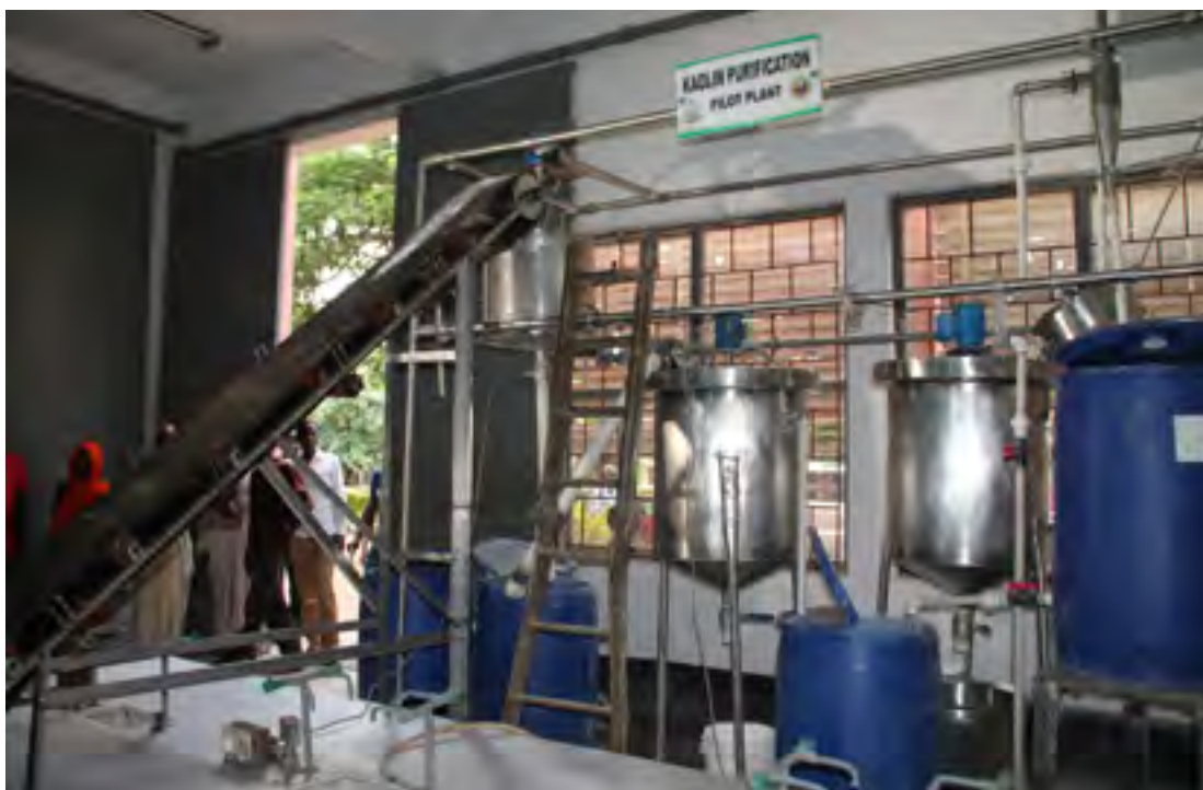
Kaolin purification pilot plant, ABU Zaria for the production of Zeolite Catalyst
